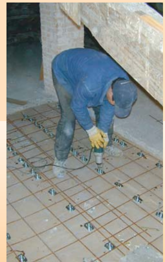
Fixing the connectors with an electrical impact wrench and a 13 mm hexagonal insert.
