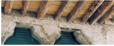
Underneath view of a floor requiring reinforcement. The well-preserved beams made static adaptation possible using this technique.
