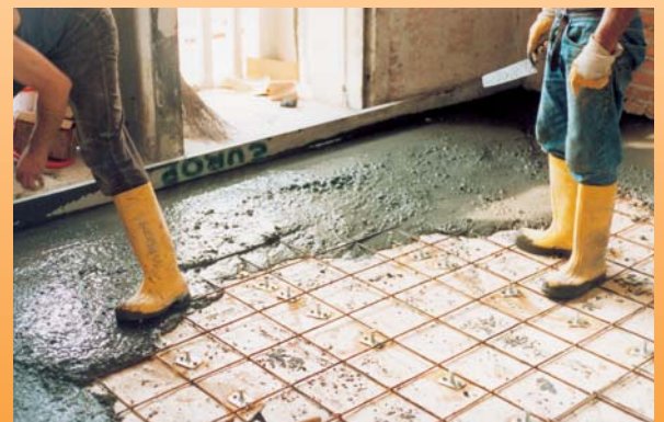
A suitable sized electro-welded mesh was inserted in the concrete. The photo shows the concrete being poured. The floors were shored beforehand.
