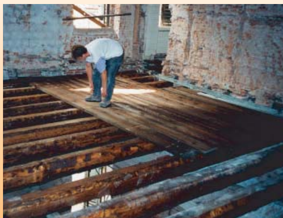
After fitting the new wooden beams in the existing holes, the boarding was laid and nailed on top.
